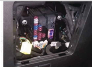
16. Get regular electricity in the fuse box
